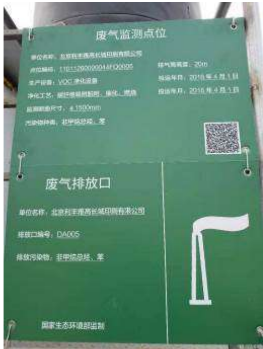
挥发性有机废气DA005排气筒
