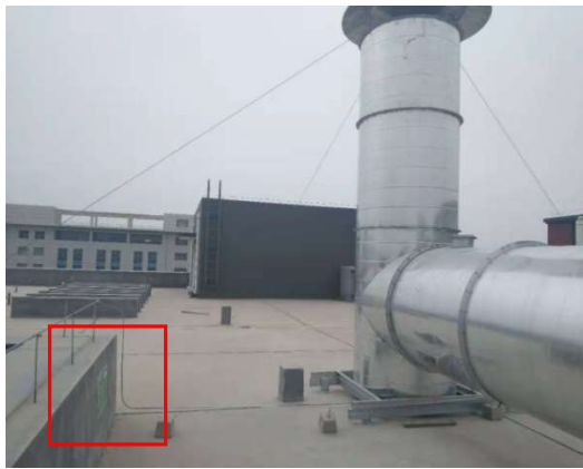
DA001 废气排气筒、排放口标识
